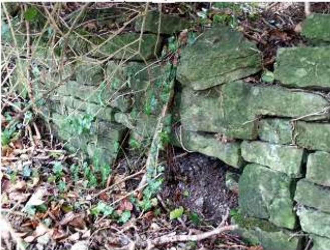
The square drain in the ha-ha wall
